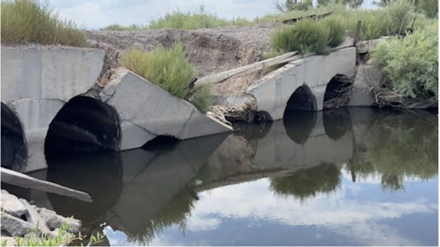
Collapsed San Luis Central RR bridge near Monte Vista, CO, August 2, 2024. ©2024 Chip
