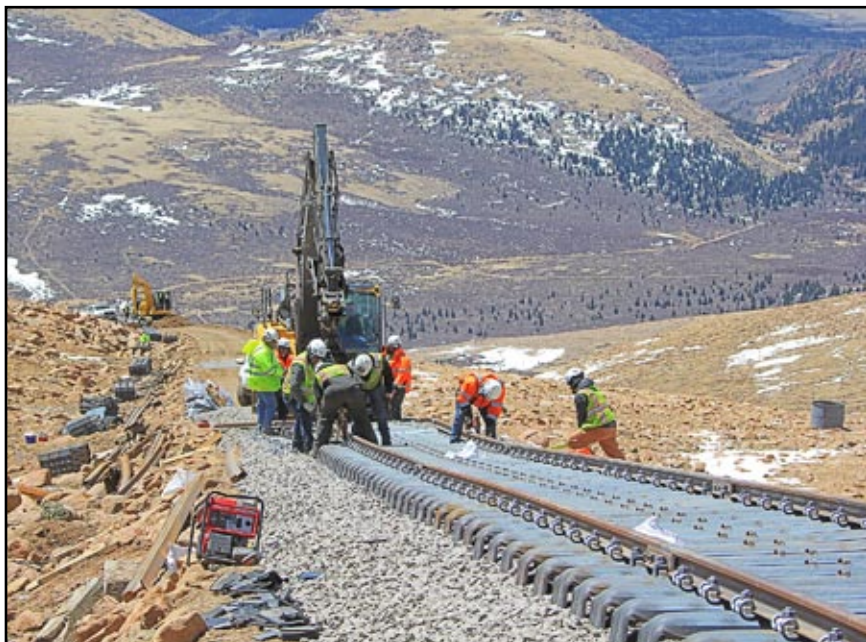
Rail is shown here being fastened to specially formed steel ties. – Photo © 2020 Dave Schaaf.
